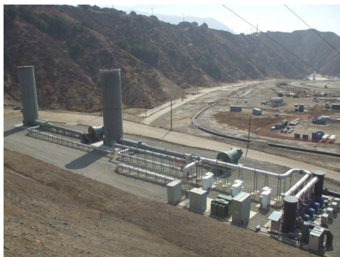
Pictured above: Flares 9 and 10 at the Sunshine Canyon Landfill. Pictured above to the right: Construction of Flare 10.
